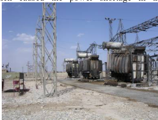
Fig.1 The 400 kV Electrical Power Transformer Station bombed by U.S. Air Force in Nasiriyya on March 22, 2003, with a carbon fiber bomb (Source: R. E. Brigety, Human Rights Watch, 2003, [4])
